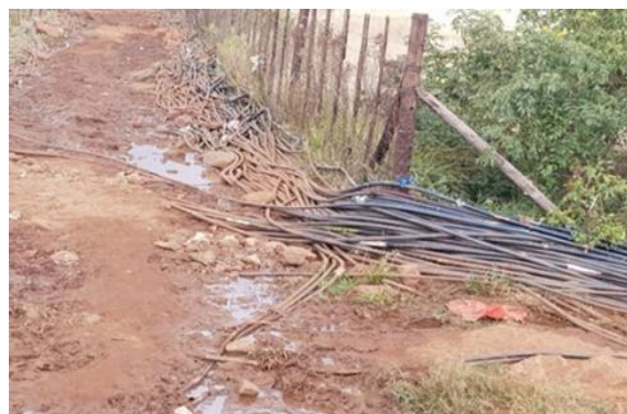
Illegal connections in Raliphaswa village Nzhelele
